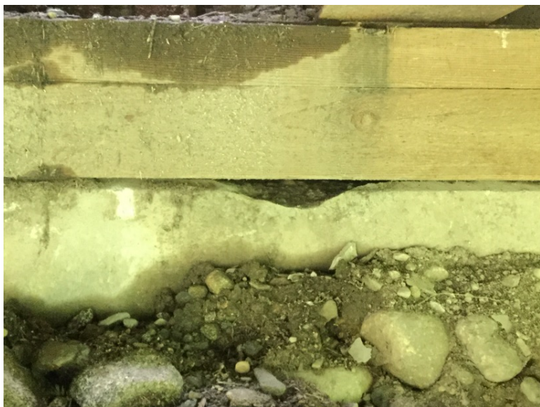
Damage noted to right bank concrete cap
