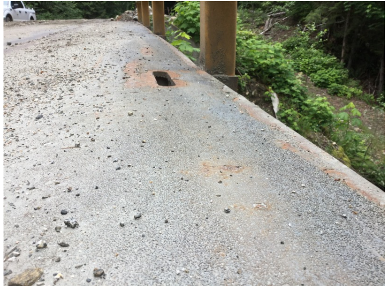
Deformation of deck plate on downstream girder
