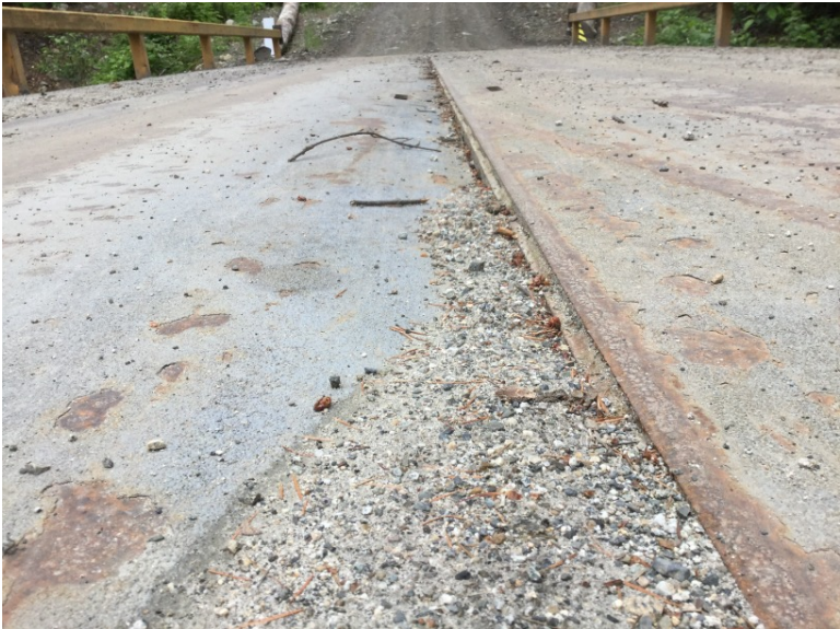
Deformation of deck plate on downstream girder
